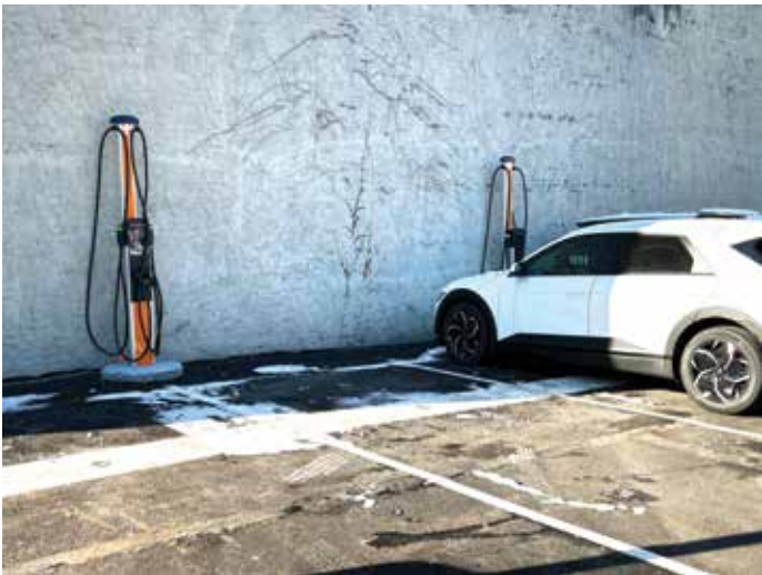
New electric vehicle charging stations.
